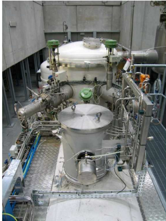
Figure 8.29: Photo of ALPI Cold Box, recently upgraded with a 3 rd turbine.
