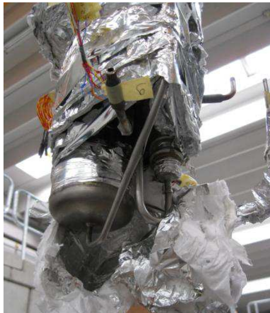
Figure 8.37: Internal purifier of ALPI refrigerator: damage, occurred in 2010 because of excessive water pollution, is visible
