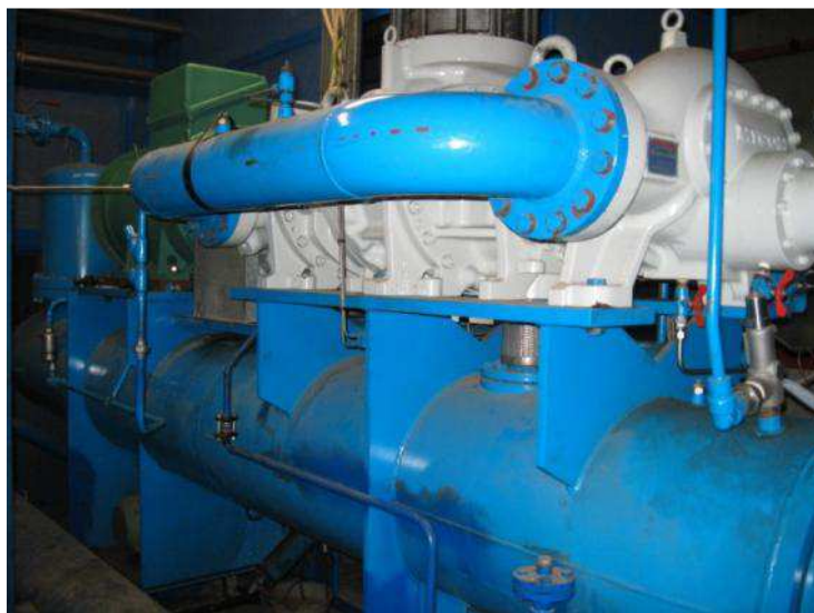
Figure 8.43: screw compressor of ALPI-SPES cryogenic plant
