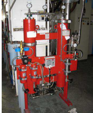
Figure 8.36: Gaseous helium dryers
