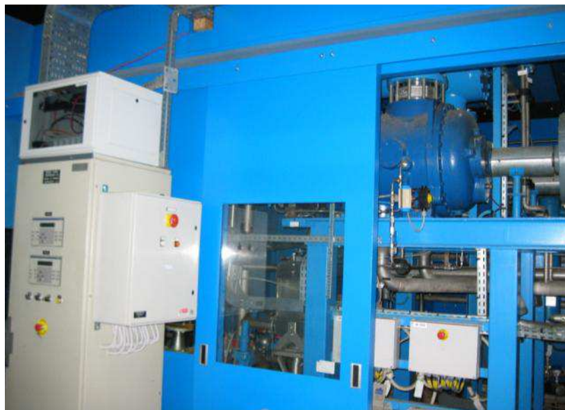
Figure 8.35: Compressor units C and D
