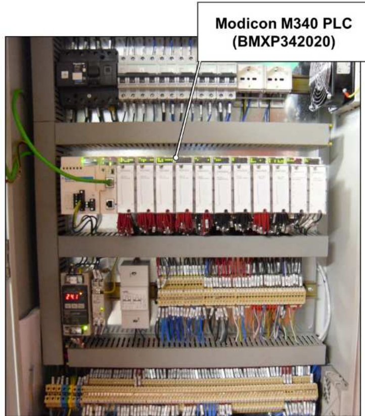
|||||: Conventional PLC used to power on and off the systems and to monitor the status of the safety control system.
